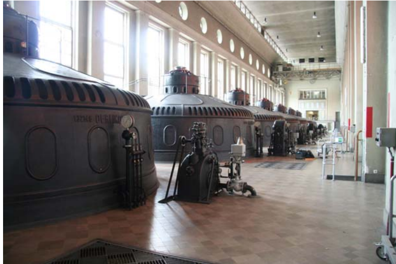
Figure 2 : View on the power house machine floor.
